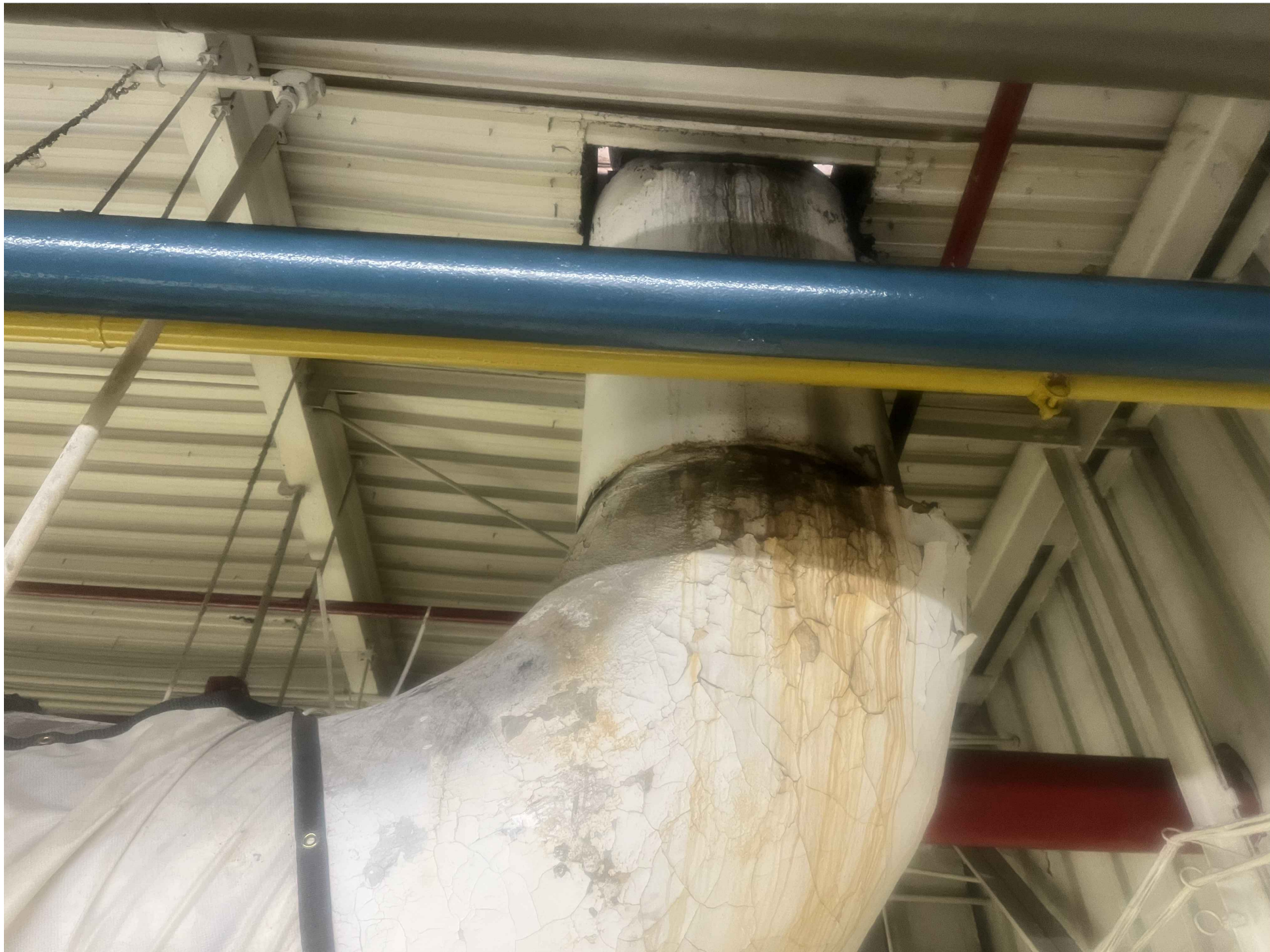
PHOTO No.01: TEST CELLS 73-84 EXHAUST
