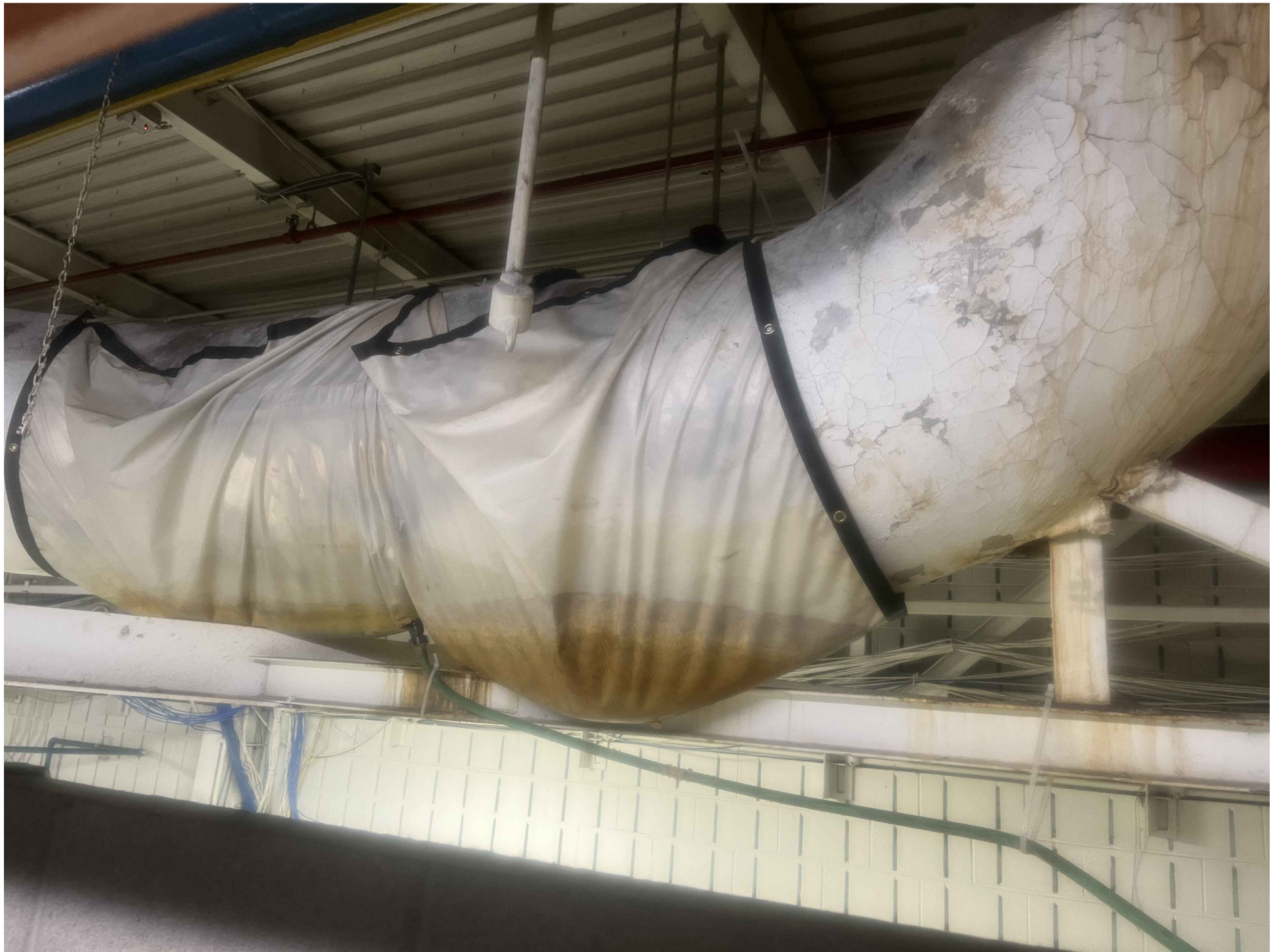
PHOTO No.02: TEST CELLS 73-84 EXHAUST
